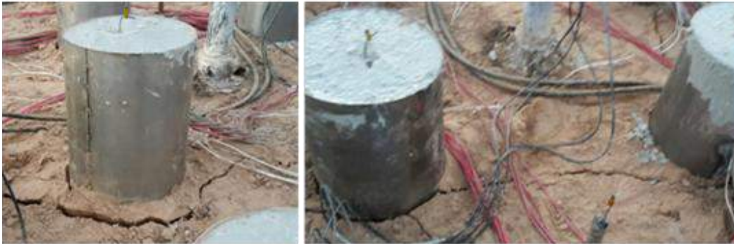
Fig. 16a Photographs of cracks in ground surface at a corner pile and at two side piles.
