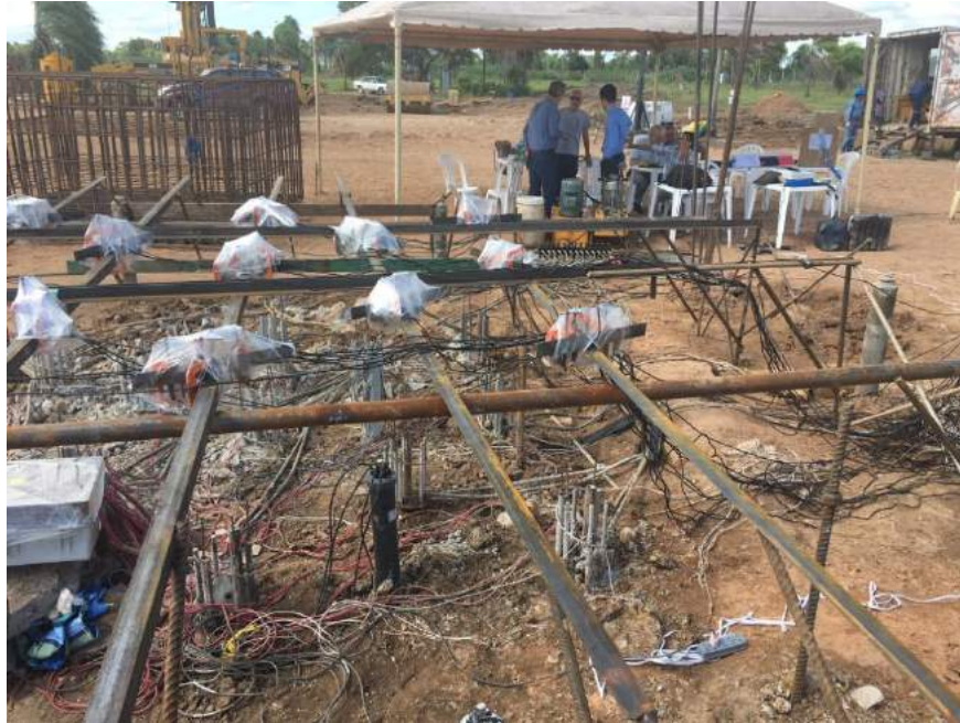
Fig. 7 Photo of frame for recording pile movements at Phase 1 test on Piles E2 - E14.
